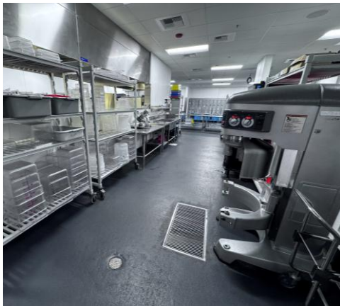
Shelving, Prep Stations, and a large mixer located in the Central Kitchen
